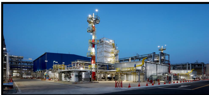
Figure 9. SGT-400 gas turbine driven CHP plant. Source: Siemens Energy website.
